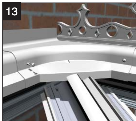
13 The joint between the full and half ridge pvc top caps is sealed by the use of a capping connector. This needs to be trimmed to suit. Bed the capping on suitable silicone and fix using the plastic rivets provided.
