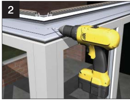
Two pilot holes already exist in the next piece of eaves beam – drill two more at 4.5mm diameter through the eaves beam and the cleat and then securely fit the four M5 x 12mm taptite screws.
