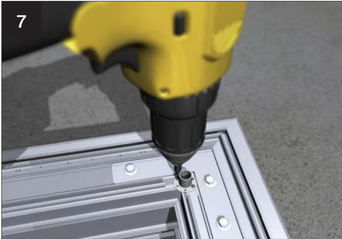
7 If supplied, fasten to each corner the tie bar drop rod fixing bracket to the underside of the pagoda eaves beam.
