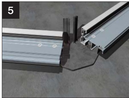
Take the second starter bar and similarly offer this onto the ridge hanger/compression plate assembly. Lift the whole "A" frame assembly and get ready to install it in its final position.
