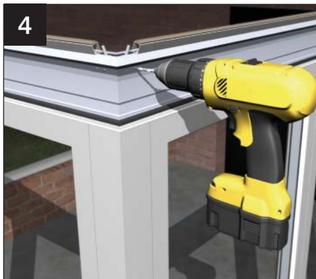
4 Using the pre-drilled pilot holes, drill two 4.5mm holes through the corner cleats.
