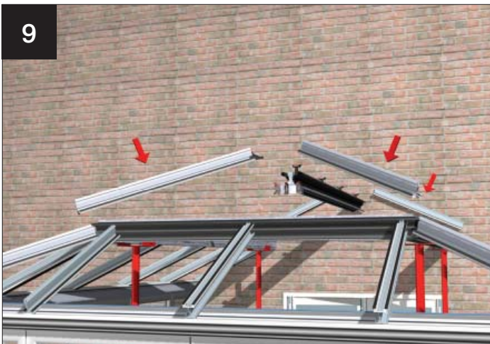
9 Using the roof location plan, build the upper roof as per section 5 of this guide
