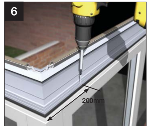
6 Securely fit the eaves beam to the frames using for example, 38mm x 4.8mm screws in the position shown. Fix down at 450 centres and within 200mm of each corner. For 60mm frames use the inner eaves extrusion line and outer line for 70mm frames. Always screw down. (Not supplied)
